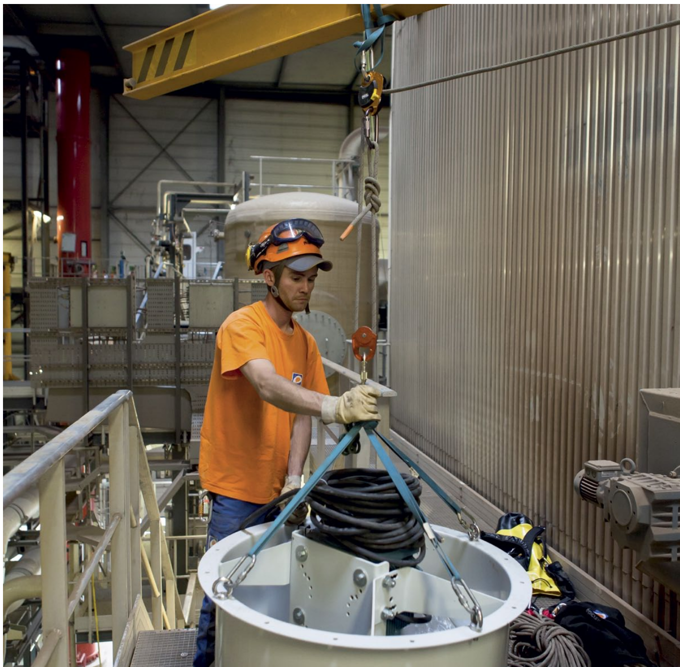
EPICURE, Usine retraitement des eaux, Pierre Benite, Rhone, France © Lafouche
